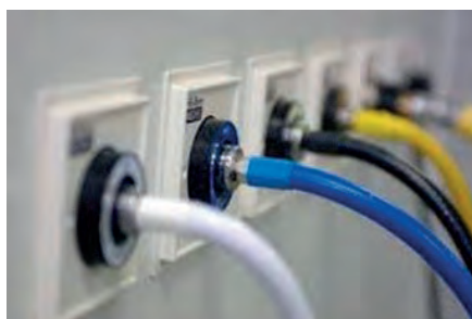
Figure 19: A set of medical gases outlets/inlets
